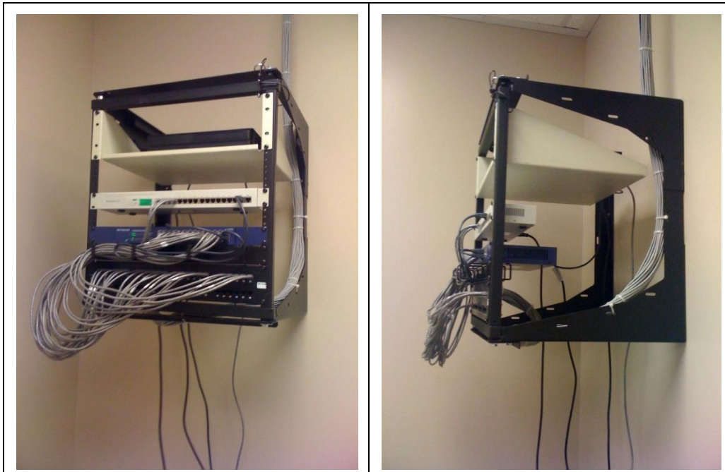
Figure 2. Example of Networking Rack
