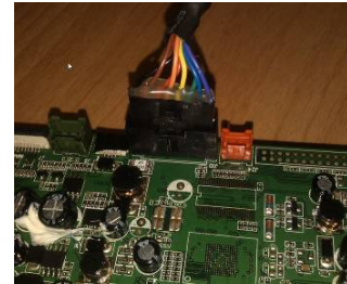
cable connection not be inserted fully
